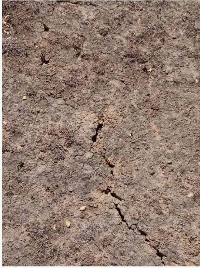
Figure 84. Surface crusting, desiccation cracks and an initial linear zone of infiltration into the soil resulting from subsurface karst solution, collapse or, most likely, suffosion.
