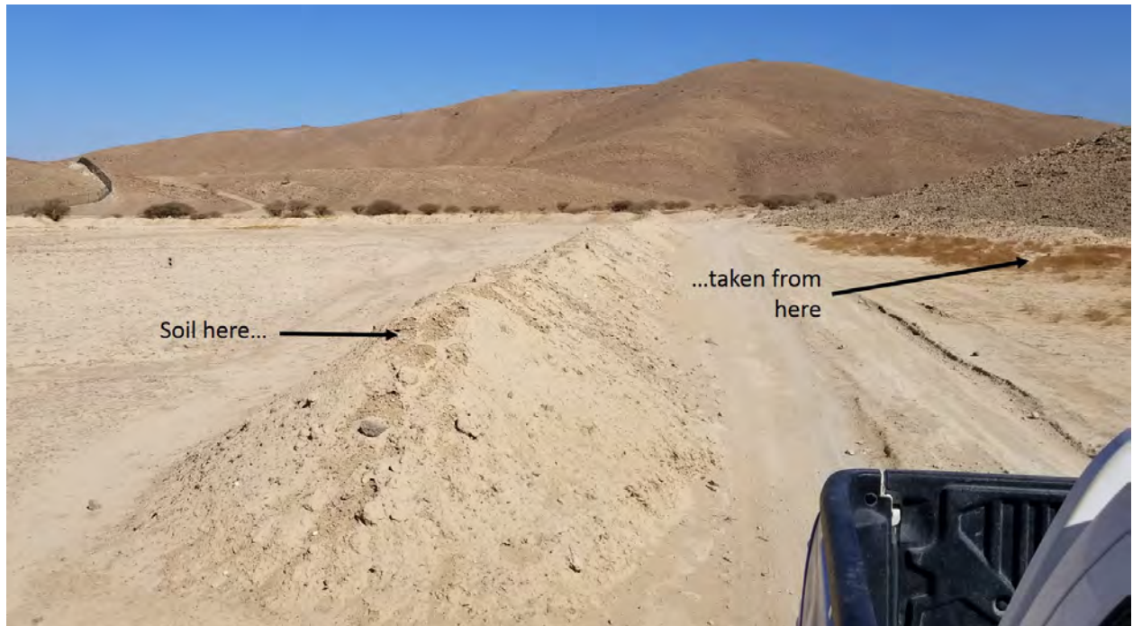
Figure 40. Bulldozing within the UNESCO site. Here the al-Qa'a football field has been surrounded by a protective bund. This bund was made from soil bulldozed from the surrounding area. This entire area should be checked for archaeological remains either exposed or damaged by these activities.
